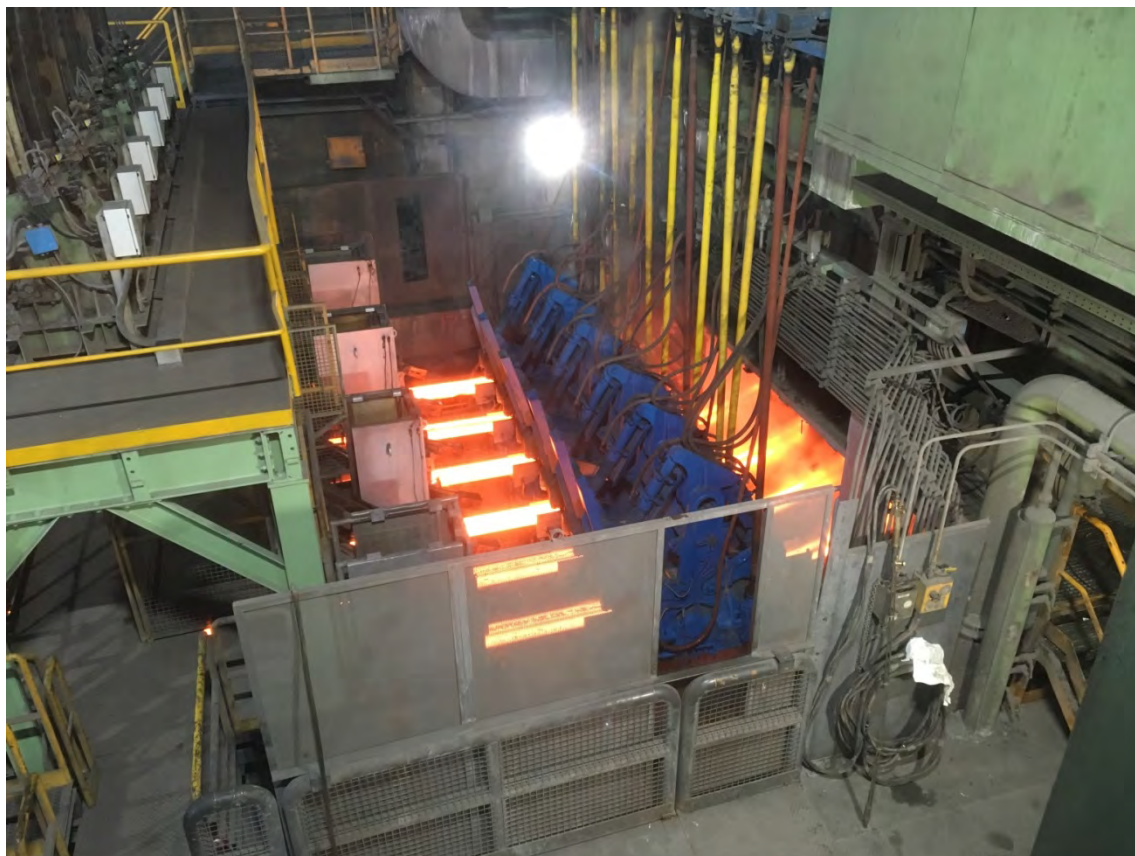
Continuous billet caster modernized by Primetals Technologies in the Lonato del Garda, Italy works of Feralpi Siderurgica
