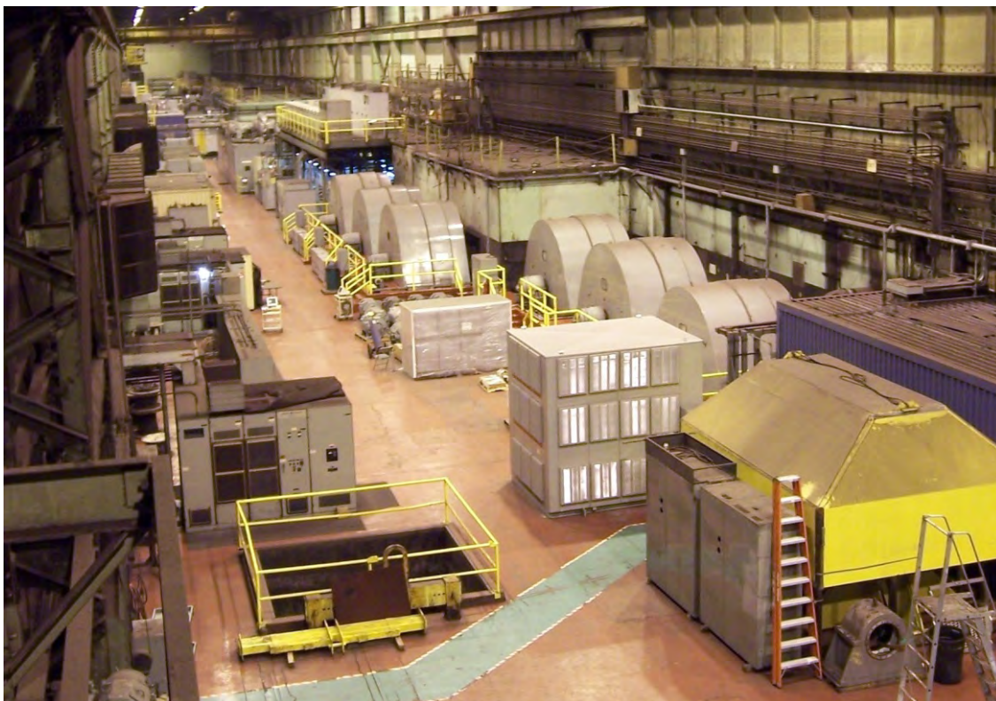
Finishing mill motor room at California Steel in Fontana, California (Photo courtesy CSI).
