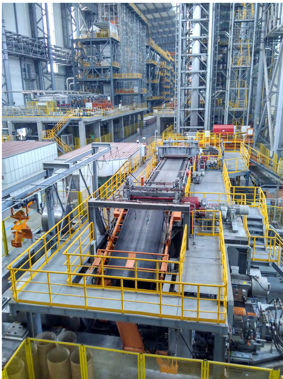
Continuous galvanizing line (CGL) from Primetals Technologies
