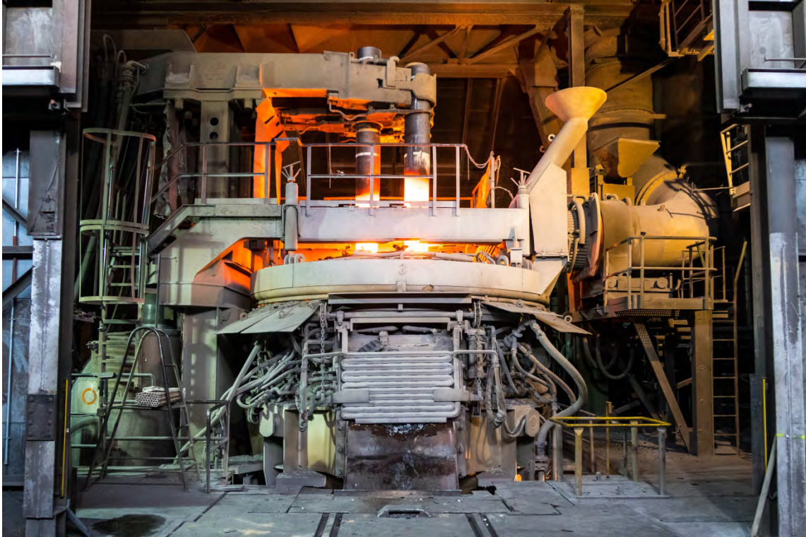
Electric arc furnace modernized by Primetals Technologies at BGH Edelstahlwerke GmbH in Freital, Germany
