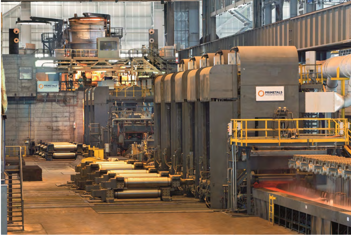
Arvedi ESP plant in operation
