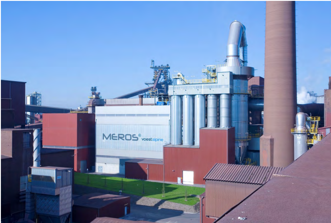
Meros plant from Primetals Technologies at voestalpine Stahl GmbH in Linz, Austria.
